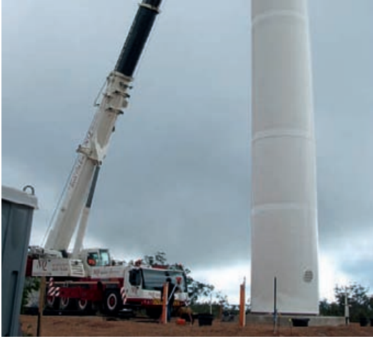
The Weather Watch Radar Tower was trucked on semi-trailers from Adelaide then assembled and raised on site.
